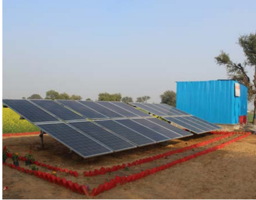
A community-based solar RO plant constructed under the Model Village Development Project in Rewari, Haryana.
