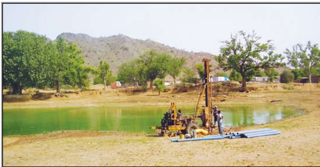
Figure 3: Recharge structure under construction at the project site, Dughera village, Behror block, Rajasthan (June, 2006)
