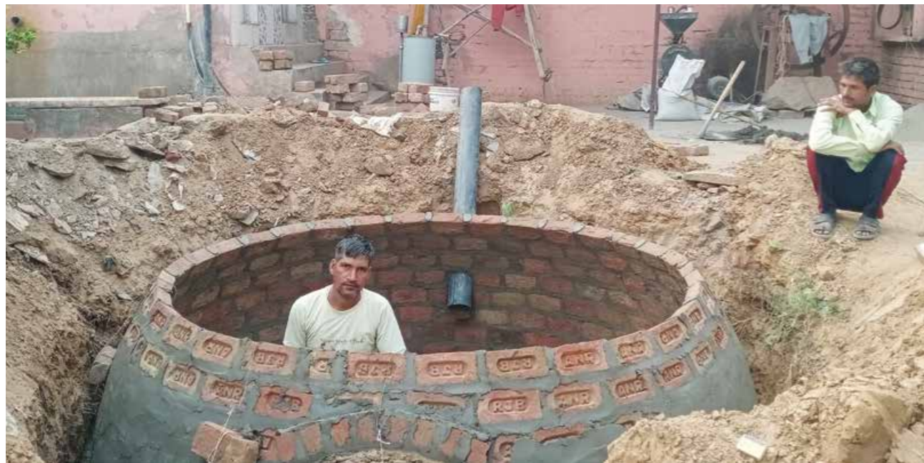
A biogas plant being constructed in Dausa Rajasthan as a part of HPPI's environmental intervention.
