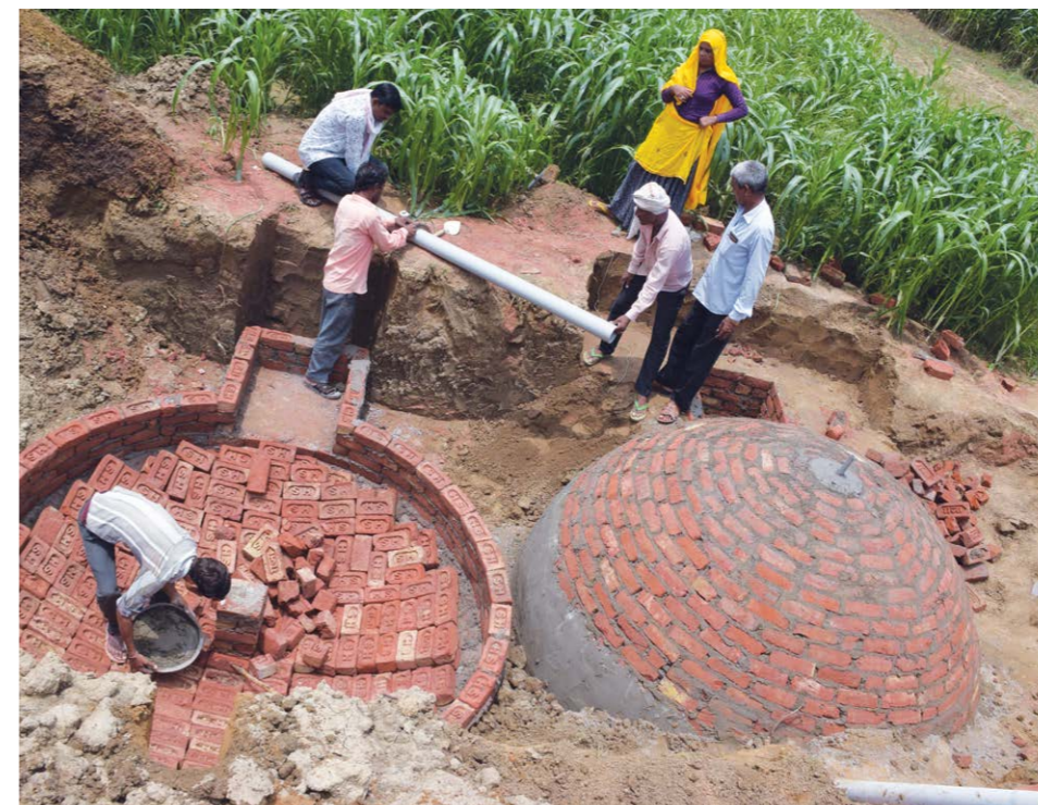
A biogas plant being constructed in Dausa, Rajasthan. Along with providing clean energy, the project is also generating employment opportunities in the area.
